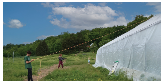
(L) High tunnel construction and (R) skinning a high tunnel. (Photos: Becky Maden, UVM Extension)
