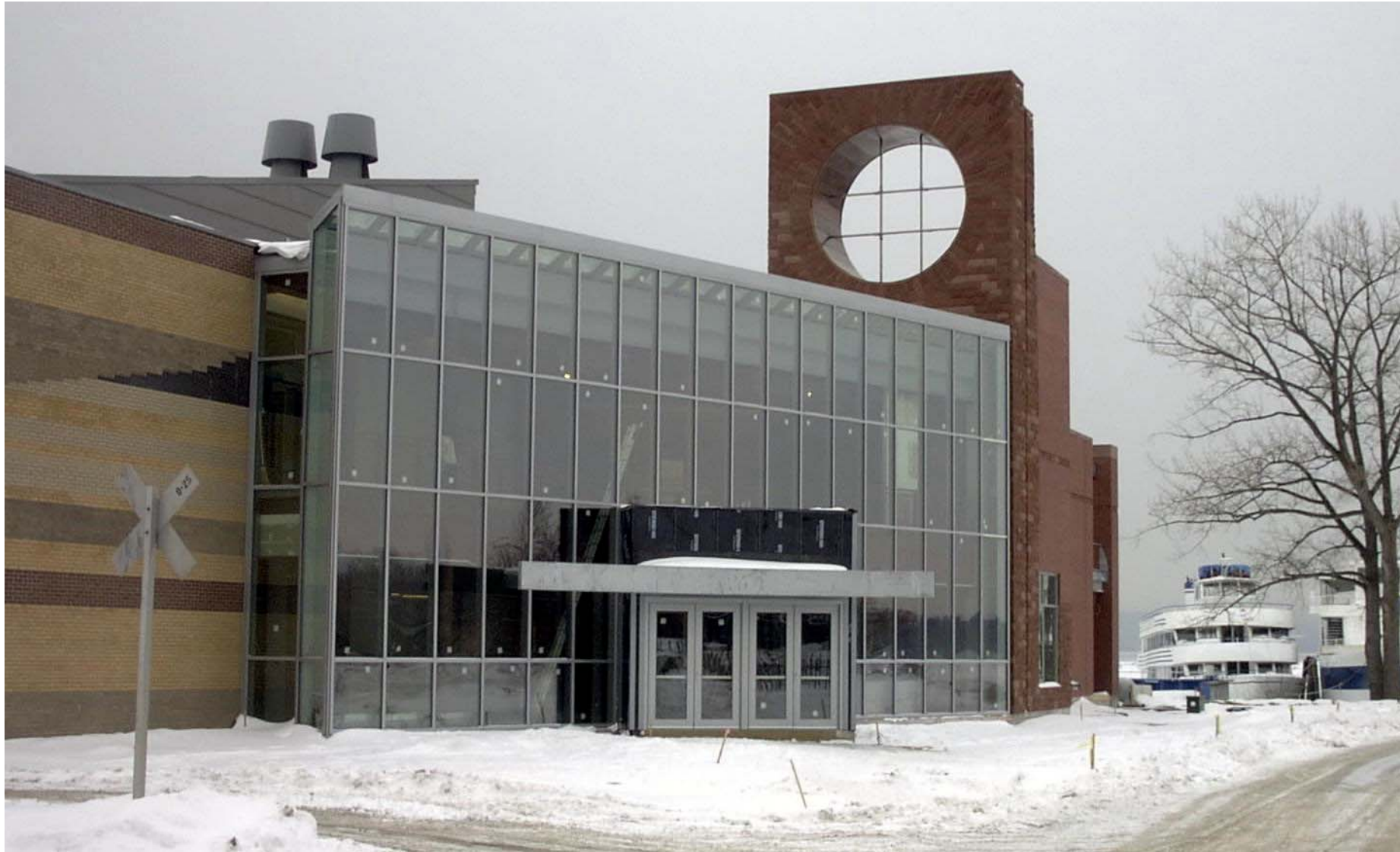
High performance curtain wall at the Leahy Center for the Lake, Burlington. Smith, Alvarez, Sienkiewicz Architects , ~2,000 sq.ft. glass curtain wall -- ~ R-4.5 !!!
