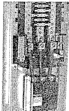
225 A QBL Main Circuit Breaker
