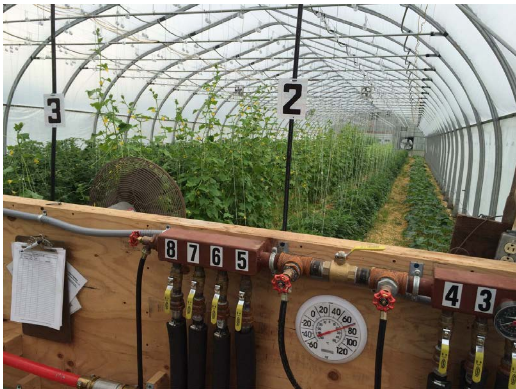
Figure 15 - Hot water distribution manifold with early cucumbers in the background at Jericho Settlers Farm (Jericho).
