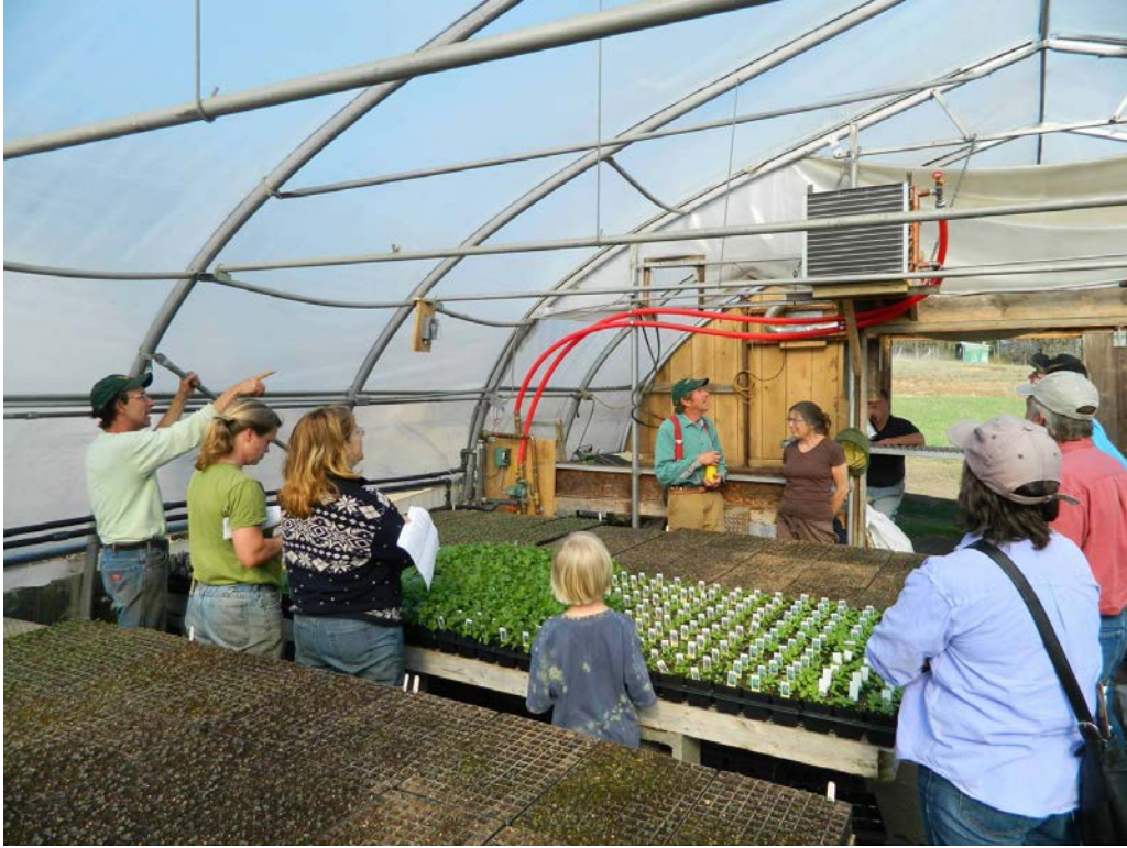
Figure 24 - Dave Marchant (Fairfax) points out the hydronic air heater in the greenhouse.
