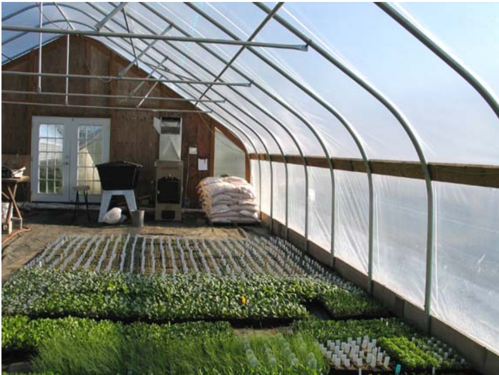
Figure 30 - LDJ shell corn/wood pellet furnace at Walker Farm (Dummerston).
