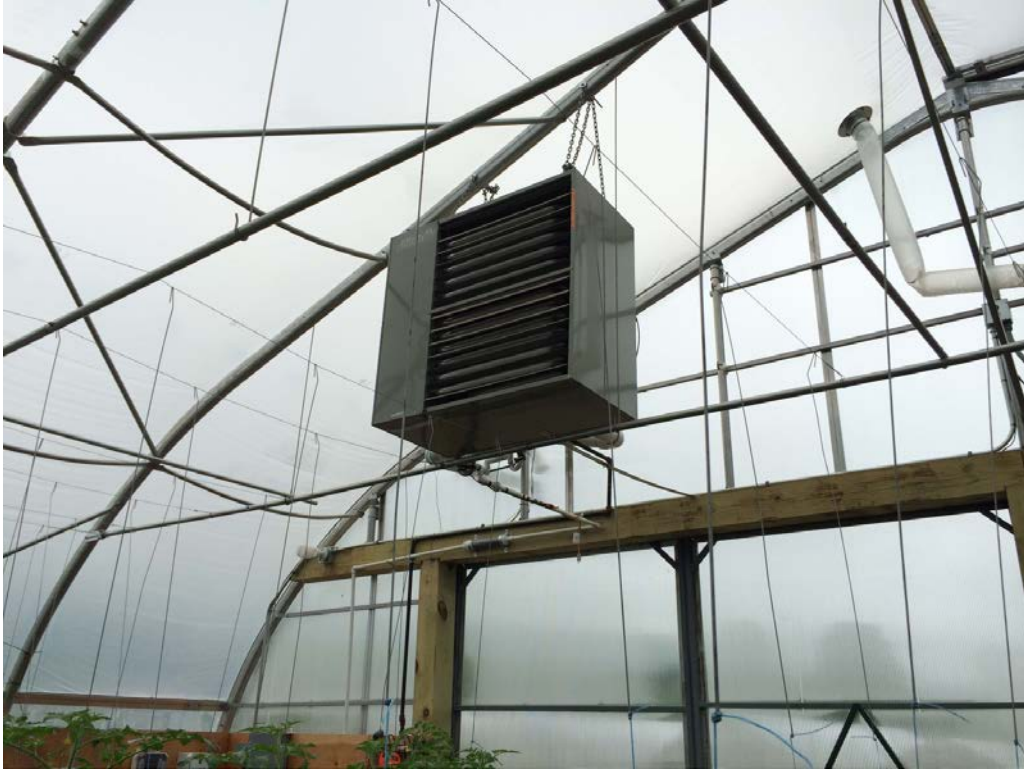
Figure 8 -Hydronic air heater (200,000 BTU/hr) at Clear Brook Farm (Shaftsbury).
