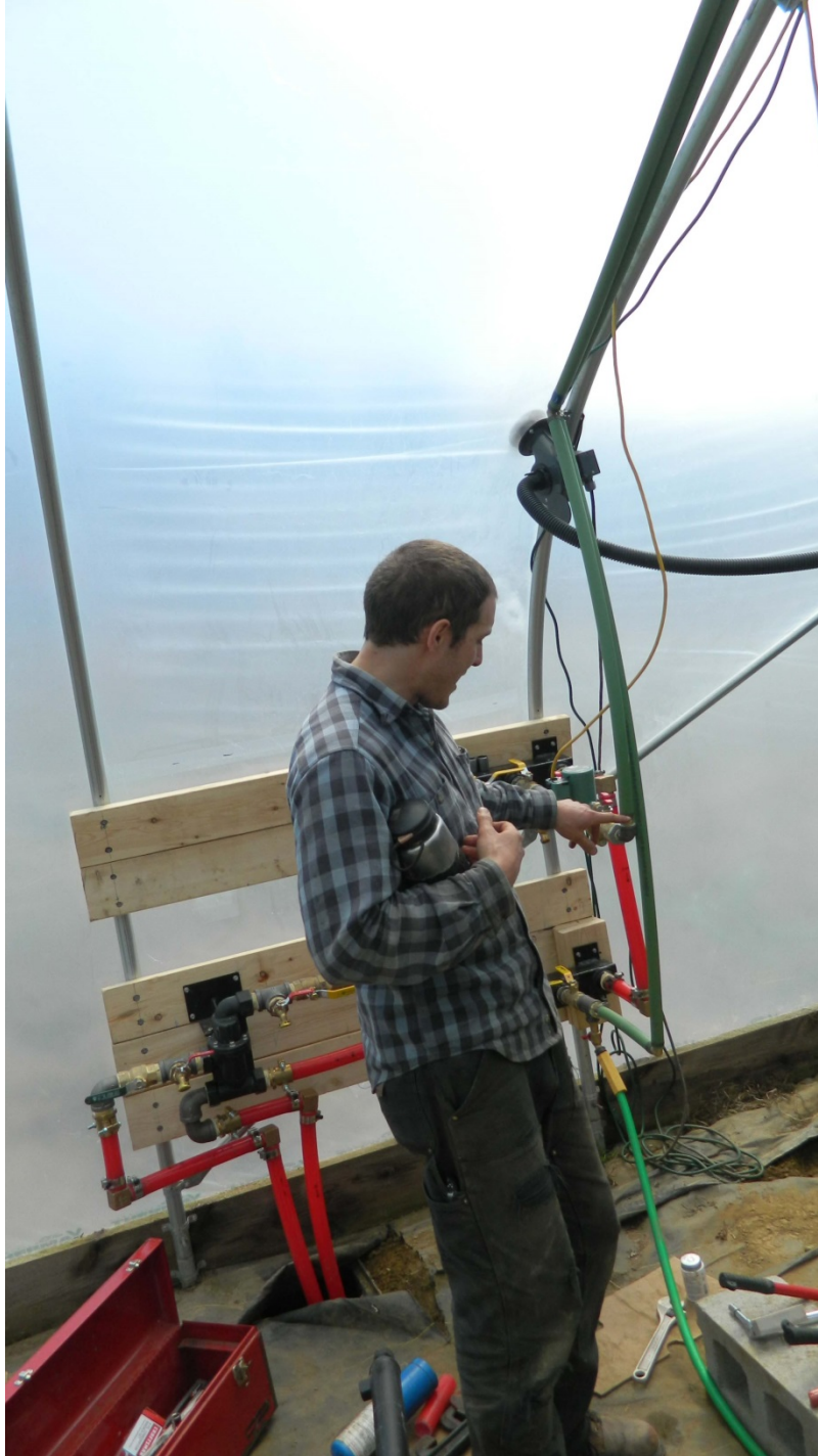
Figure 4 - Justin Rich, Burnt Rock Farm (Huntington), walking through the manifold plumbing inside the greenhouse.
