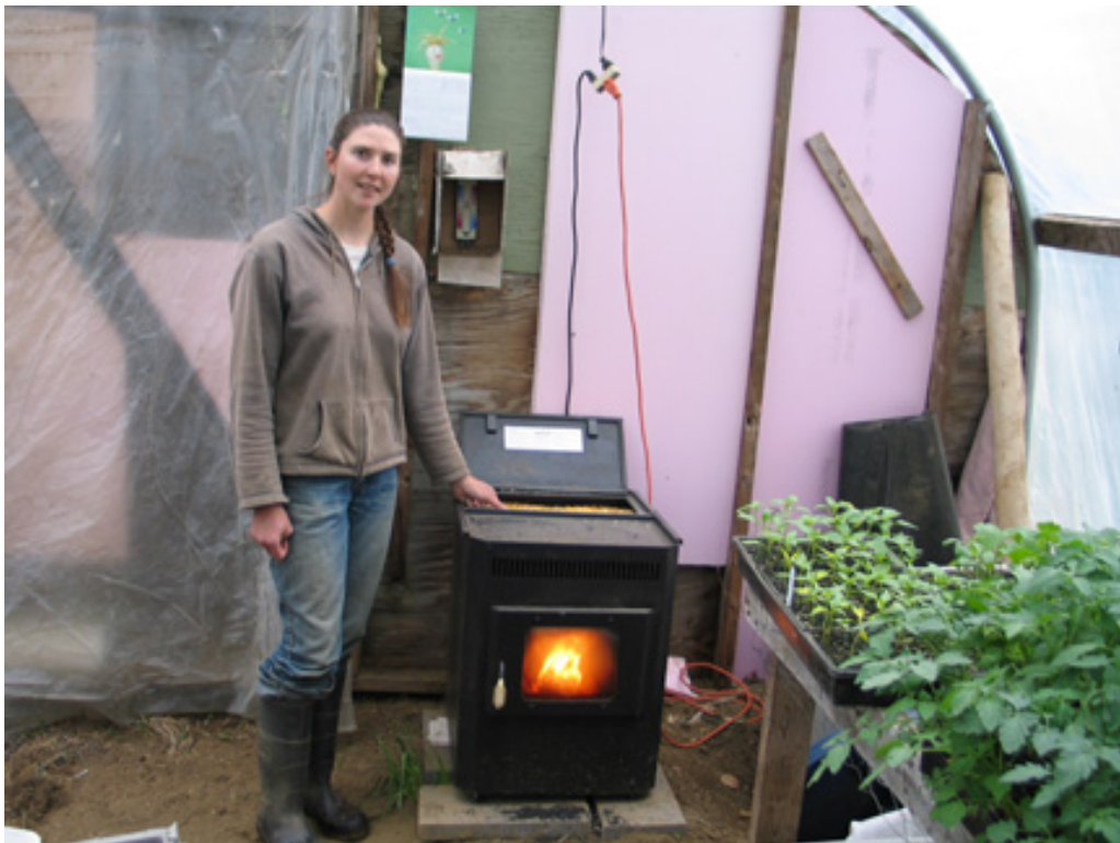
Figure 11 - Elizabeth Wood, New Leaf CSA, with Amaizblaze 2100 (30,000 BTU/hr) pellet stove used to heat a very small greenhouse for early seedling production.
