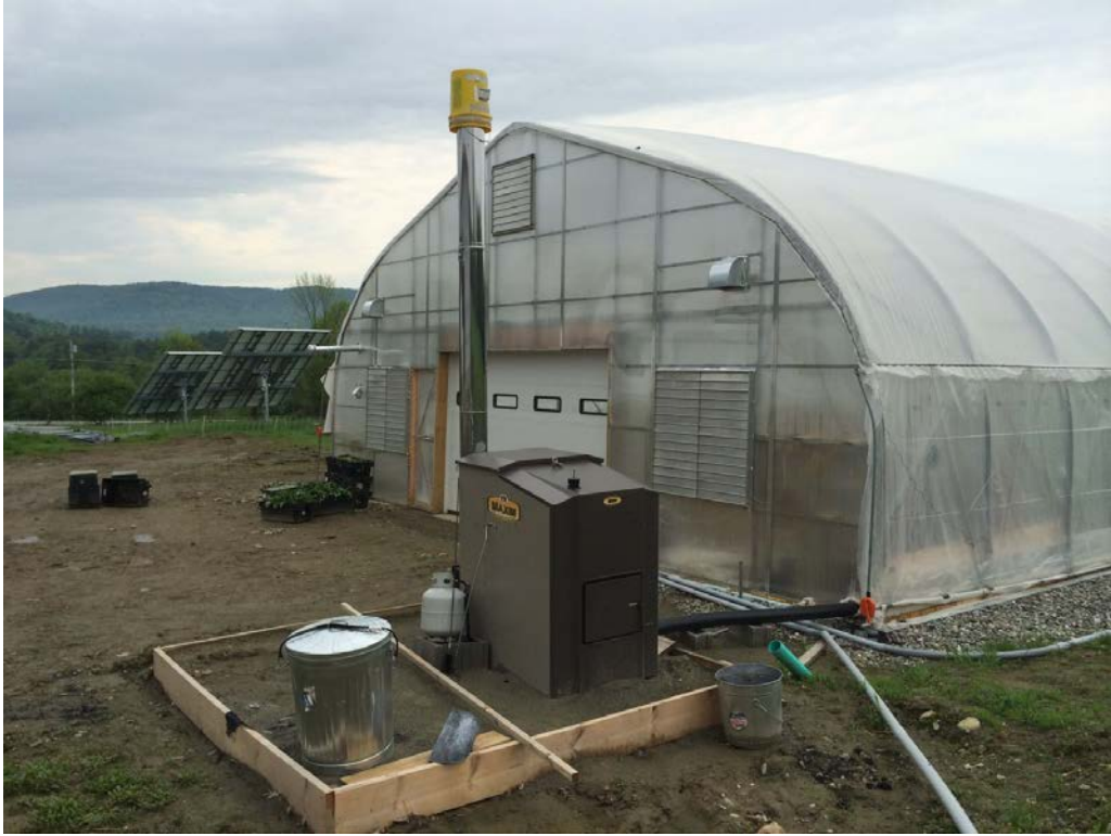
Figure 16 - A nearly completed Maxim 250 outdoor biomass boiler at Jericho Settlers Farm (Jericho).
