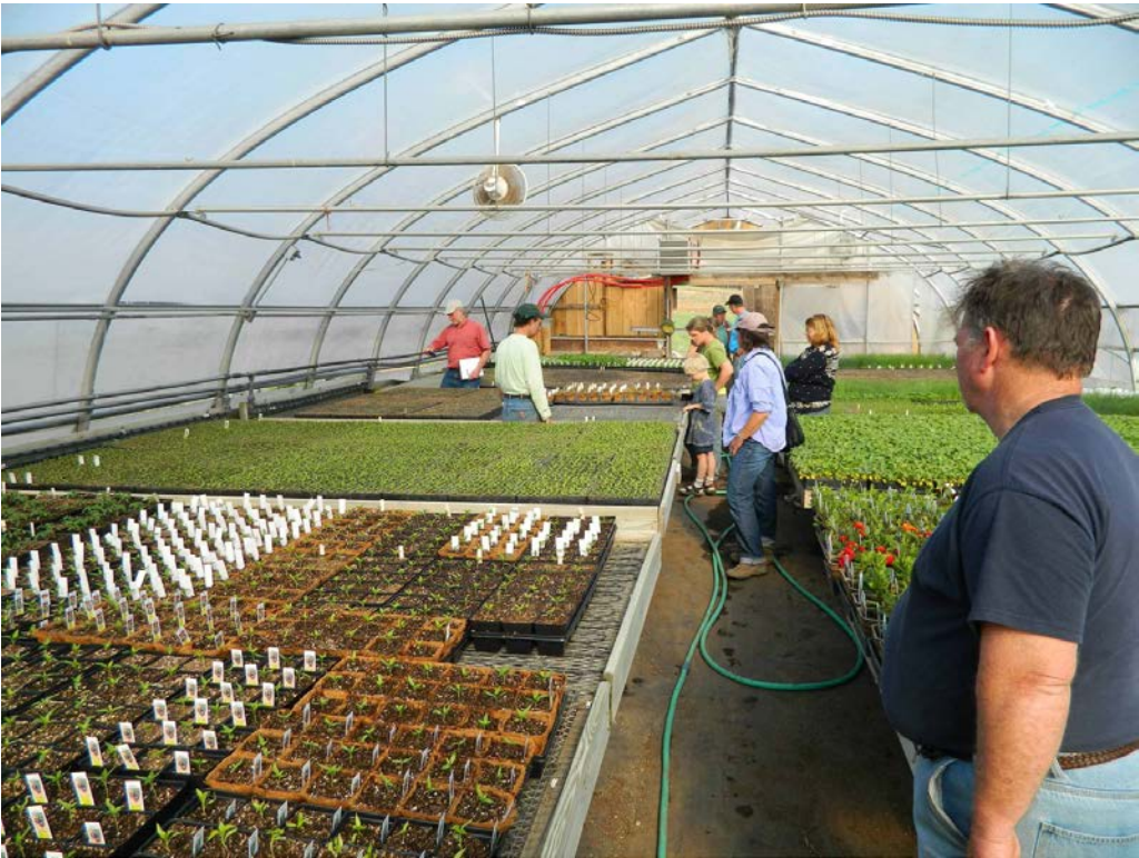
Figure 21 - Dave Marchant (Fairfax) at a later twilight meeting showing bench heating mat heated with hot water from the Maxim 250 outdoor boiler. A hydronic air heater, also fueled by the Maxim, is visible on the far end of the greenhouse.
