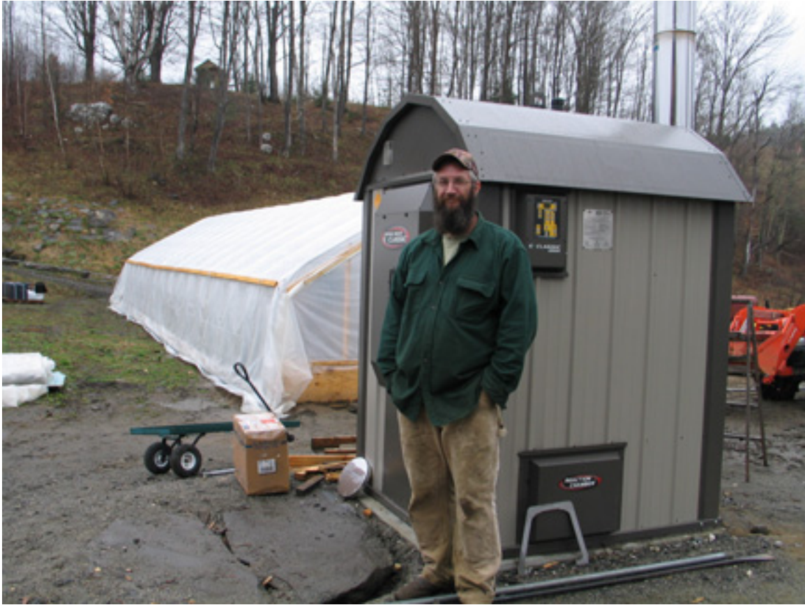
Figure 26 - Paul Betz with Central Boiler eClassic 2300 cord wood boiler, used to heat two greenhouses (Woodbury).
