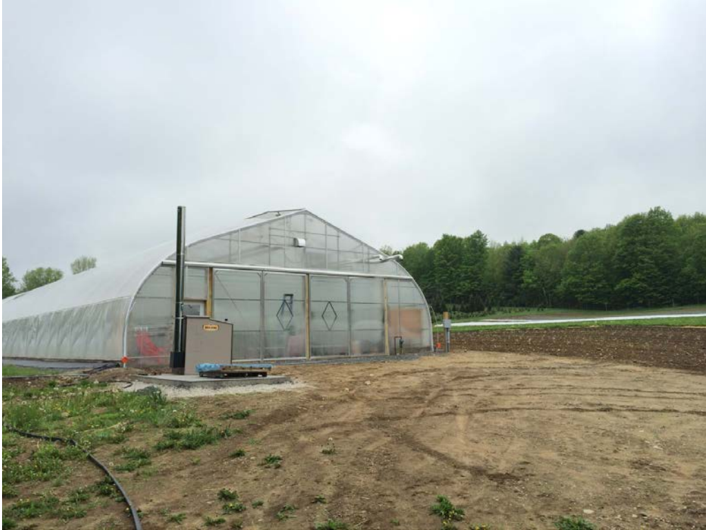
Figure 10 - Maxim 250 outdoor wood pellet/shell corn hot water boiler at Clear Brook Farm (Shaftsbury).
