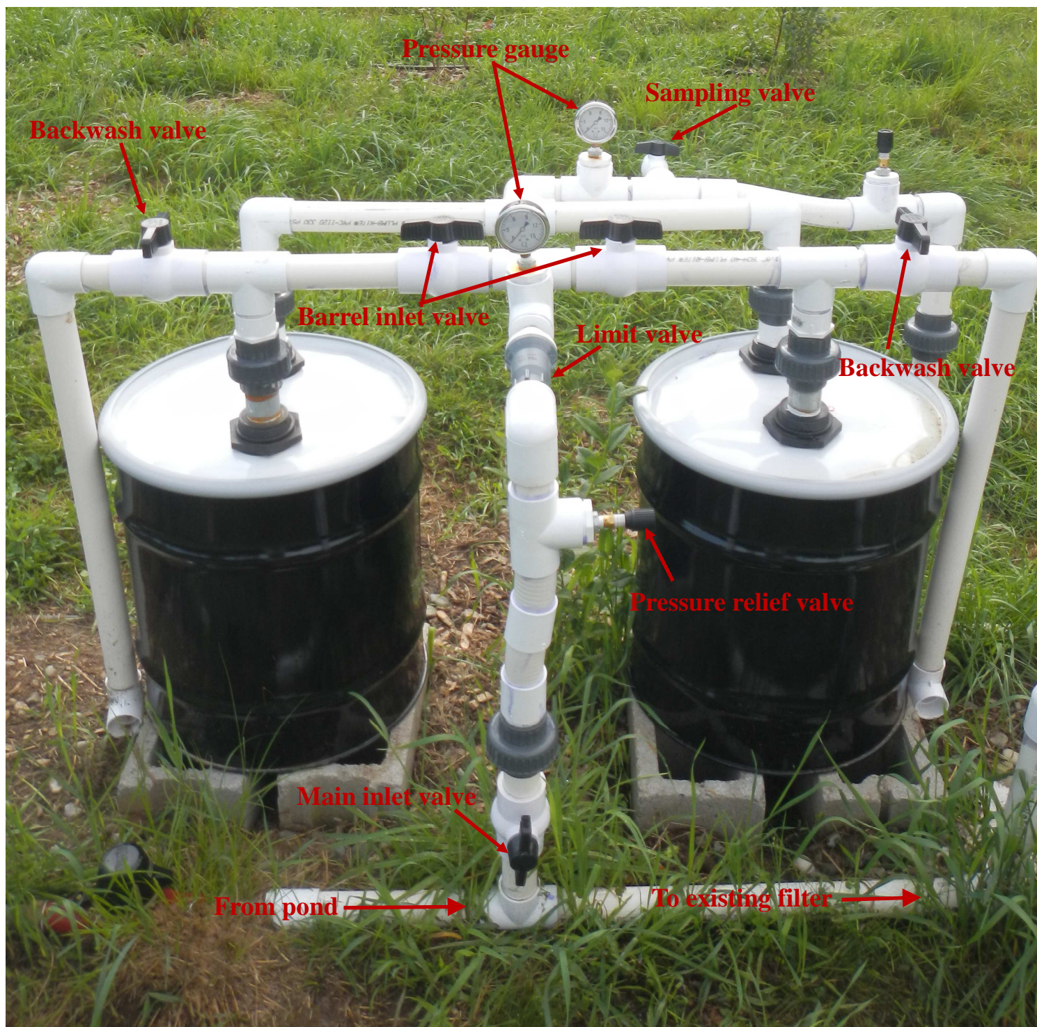
Figure 7. Front view of sand filter system with various components identified. Note: Sampling valve and pressure relief valves were for evaluation only, they are not required if appropriate limit valve is installed.
