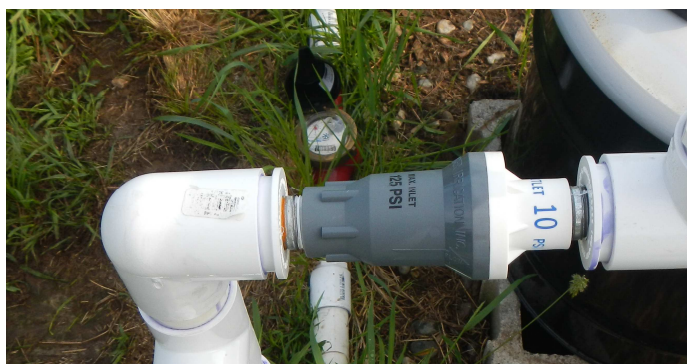
Figure 4. Limit valve on inlet line.
