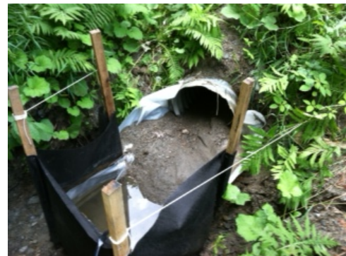
Figure 1: Plastic and filter fabric silt fence, installed out culvert outfall, with bulk sample collected after storm event in summer 2012
