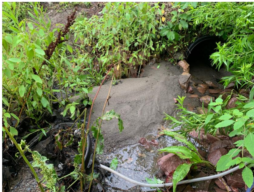
Figure 50. The Fairview Drive culvert had significant sediment accumulation during peak stormflow. This was often significant enough to displace the Thel-mar weir and disrupt water level readings.
