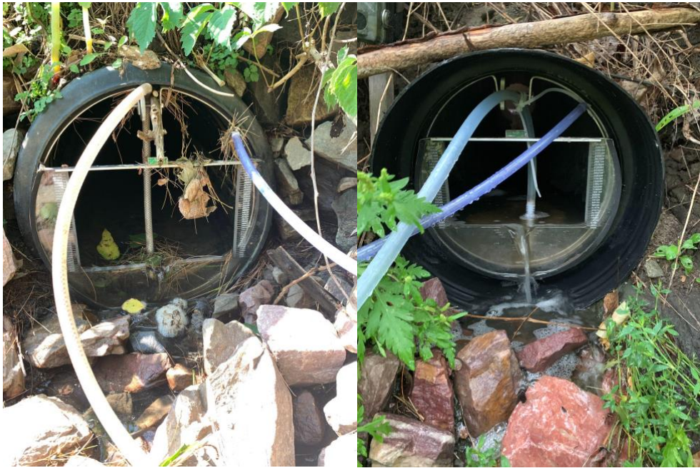
Figure 8. Thel-Mar weirs were installed at the two inlet culverts at the Fairview Wetland. Fairview Drive culvert is on the left, and Route 15 culvert on the right.
