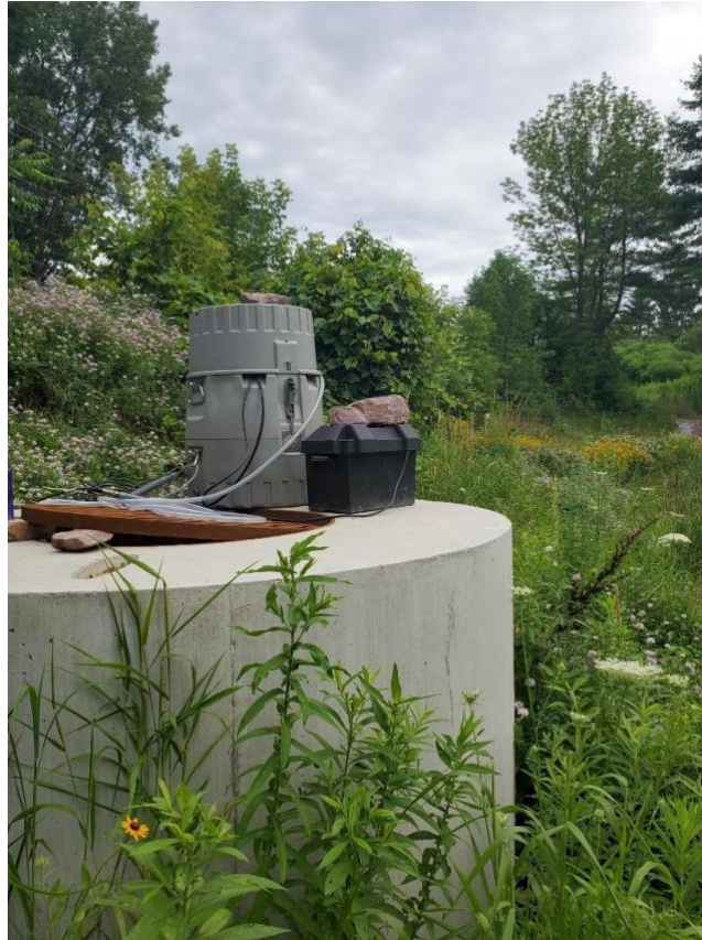
Figure 5. Example of the ISCO set up at the Fairview Outlet with a battery box adjacent.
