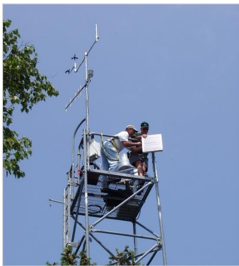
Figure 11. Meteorological monitoring equipment installed on Diamond Island in Lake Champlain.
