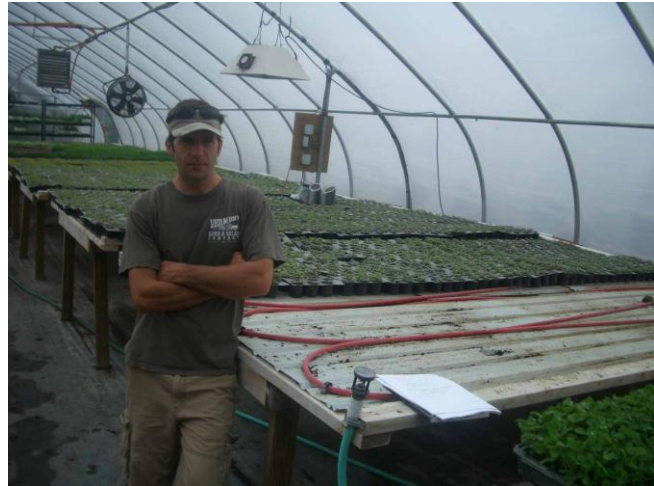
Jared in front of one of his home-made bench heaters made with salvaged metal roofing and PEX tubing.
